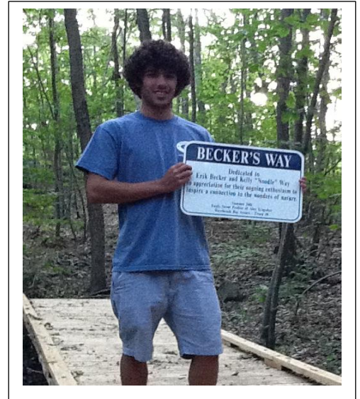
Pic: Alex standing on his Eagle Scout project, a bridge he constructed for Bushy Hill
